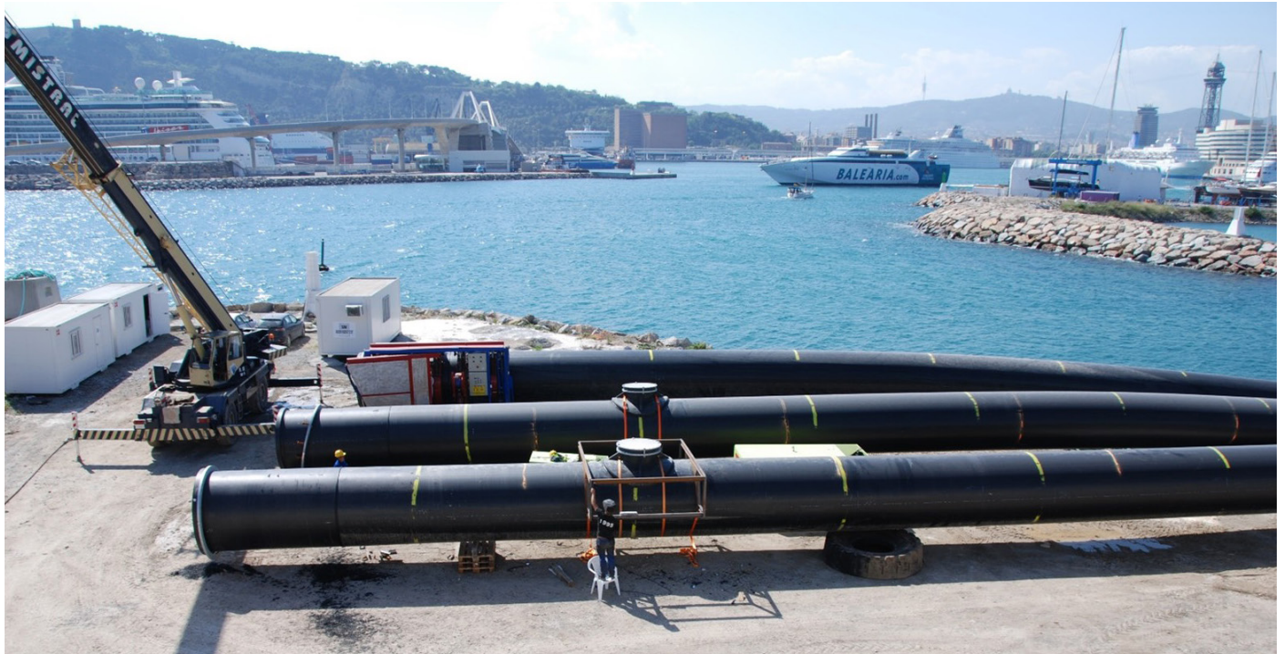
Pipe preparation for stub-end welding prior to delivery (Tangiers) and manhole installation (Barcelona)
